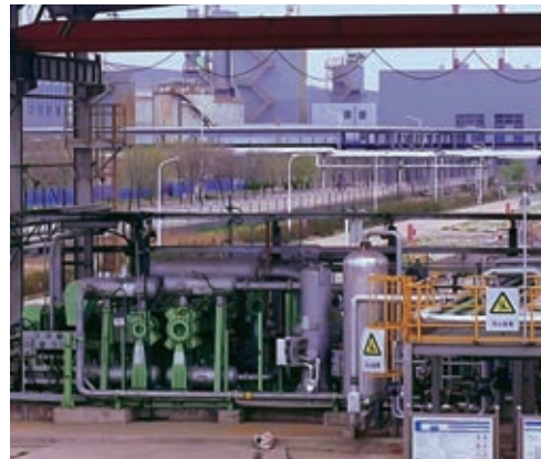
唐山旭陽化工有限公司PSA裝置 PSA Plant of Tangshan Risun Chemical Limited
