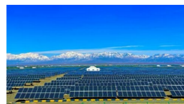
Shichengzi Photovoltaic Power Station
