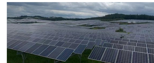
Equipment Lease-back Project of Photovoltaic Power Generation for Shilin Yundiantou New Energy Development Co. Ltd.
