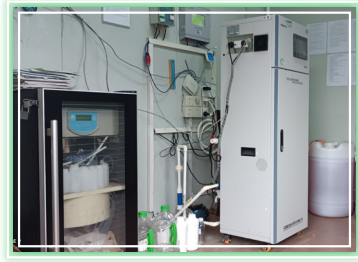
Sewage online monitors
