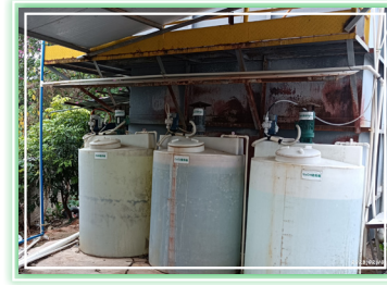
Sewage phosphorus removal equipment
