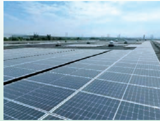
Photovoltaic Power Generating Facility on Plants Site Installed
