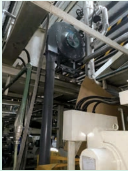
High-Efficiency Fan Upgraded
