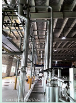
Steam Recycling System Installed
