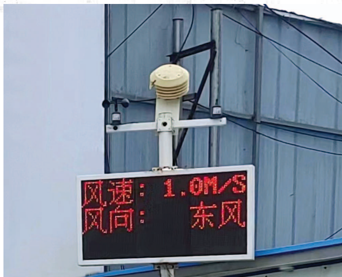
Air quality monitoring system installed on site
