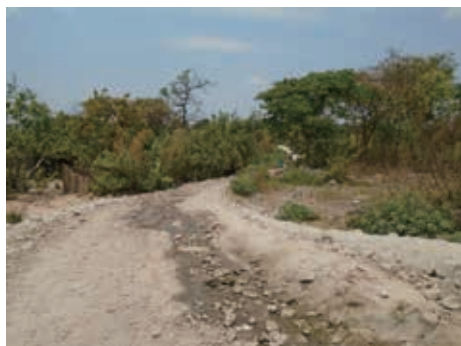
Road erosion status
