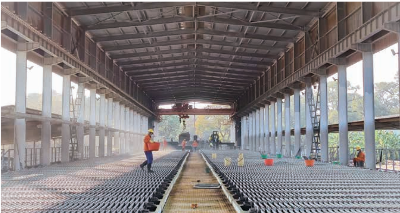
CNMC Huachin Mabende extraction electrowinning workshop
