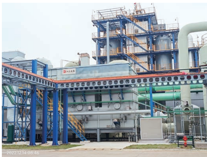
Three-chamber RTO facilities
