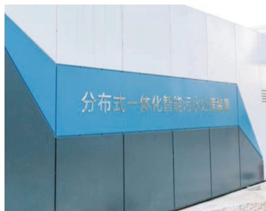
Integrated intelligent sewage treatment unit in Zhoupu Park
