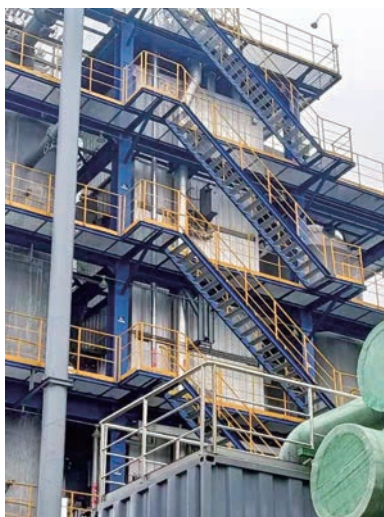
Waste liquid incinerator with exhaust heat boiler
