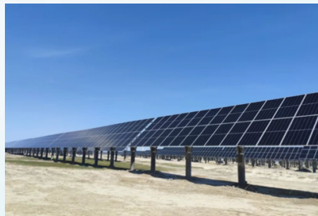
Photovoltaic project of Technologies & Engineering Company
