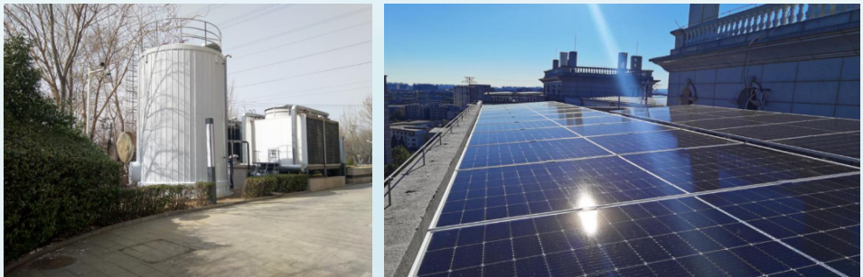
The Energy Storage and Energy-Saving Cooling System Photovoltaic Systems on Roofs and Carports
