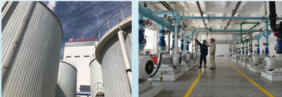
"Low Temperature Multiple Effect Flash Evaporation + Rotary Atomization Drying" combination engineering project site
