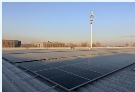
Yankai Electric distributed photovoltaic project
