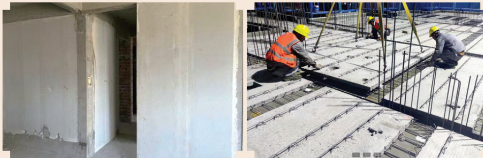
Precast lamination process (PC) and autoclaved aerated concrete wall panel process (ALC)
