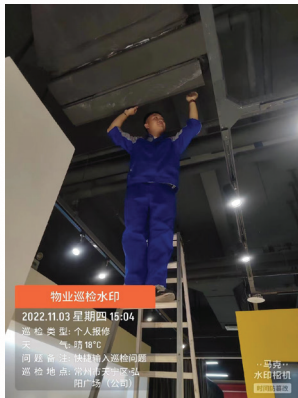
Cleaning and maintaining air conditioners for tenants free of charge 免費幫商戶空調清洗保養
