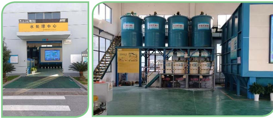
Wastewater treatment facility 廢水處理設施
