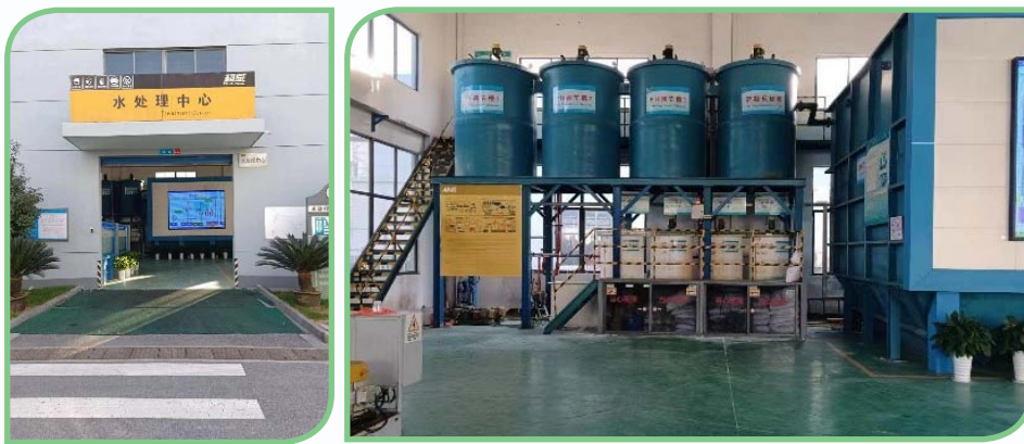
Wastewater treatment facility 廢水處理設施
