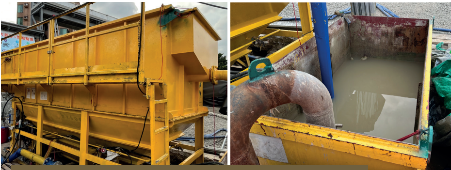
Water undergoes preliminary sedimentation in sedimentation tanks
