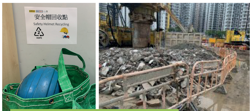
Examples of designated areas for recycling in construction sites (left: safety helmets, right: inert C&D waste)
