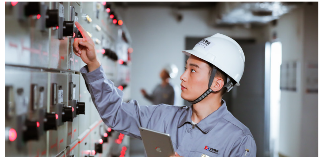
Inspection Rounds of Power Distribution Room
