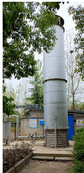
> The replaced new technology fan-less extraction torch
