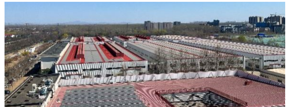
> Distributed photovoltaic panels
