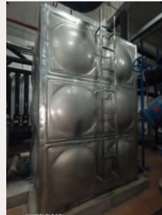
Air conditioning waste heat recovery tank
