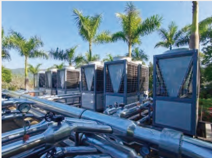
Gas to electricity equipment operation
