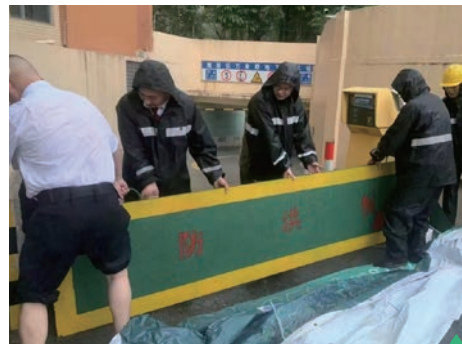
Dam anti-backfilling in rainstorm
