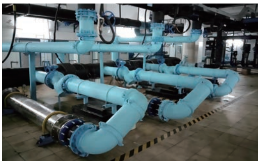
Water pump set after transformation
