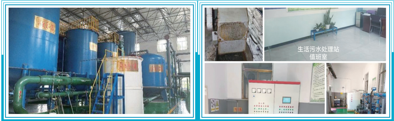
Picture: Mine water treatment equipment (left) Domestic sewage treatment station (right) 圖：礦井水處理裝置圖(左)：生活污水處理站(右)
