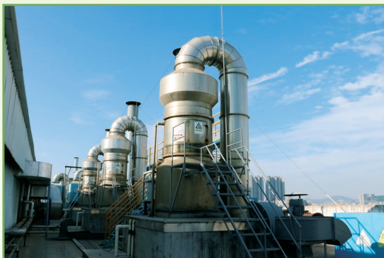
Hazardous waste treatment device in a factory 廠區危廢處理裝置
