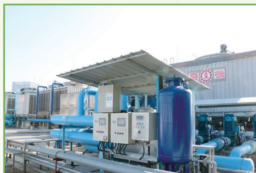
Closed circulation cooling tower 封閉式循環冷卻水塔
