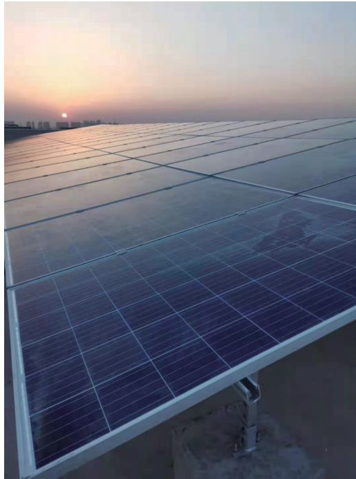
Installation of solar panels on the roof of buildings to supply hot water for the top 5-7 floors of the building. 在樓宇屋頂安裝太陽能電池板，為樓宇頂部5至7層提供熱水。
