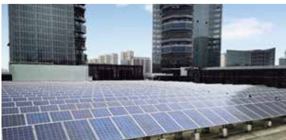
PV power generation system of Ningbo Mixc
