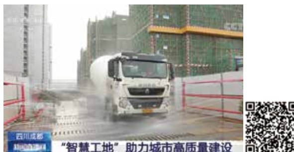
CCTV News reports the construction of smart construction site platform and EHS management of The Times City project of CR Land
