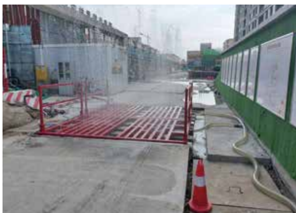
Reusing the water in the sewage treatment tank to wash muds off vehicles
