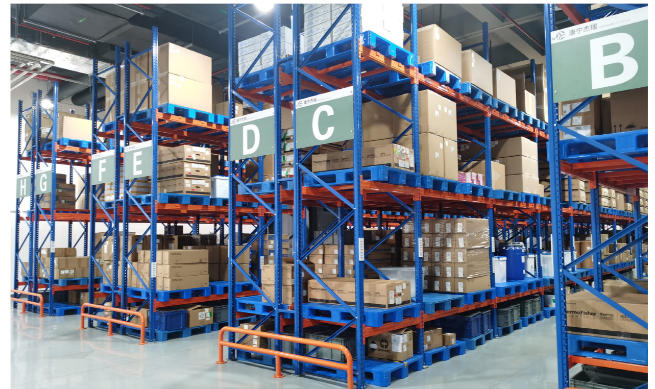
Management Project of Air Conditioning in the Normal Temperature Warehouse of Factory
