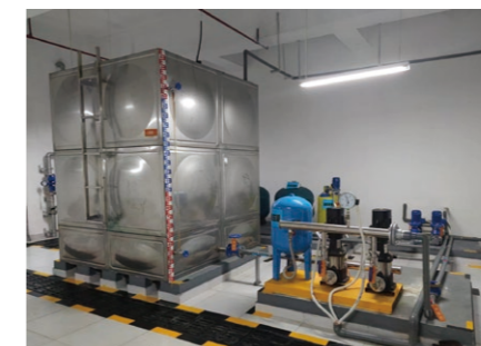
Partial picture of rainwater recycling system
