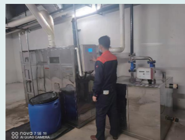
The Worker is Adjusting the Operation Time of the Oil Isolation Treatment Equipment
