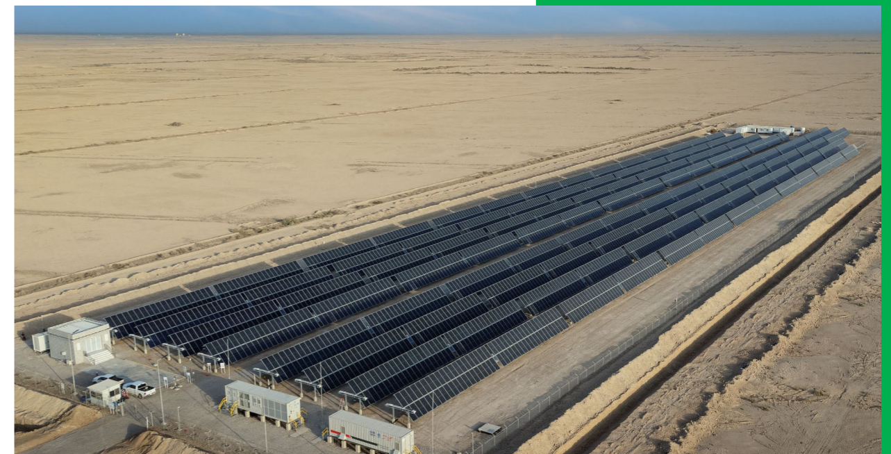
The Solar Power Plant at KEBL
