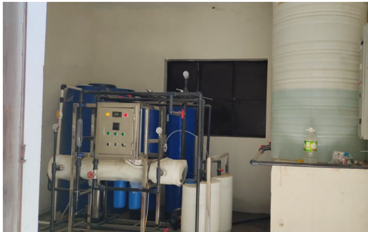
Solar Powered Reverse Osmosis Water Treatment Plants Installed for Local Communities
