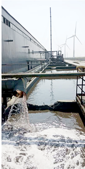
Circulating pool 循環水池
