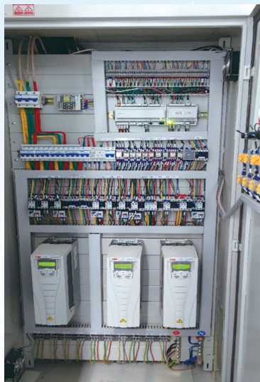
Laboratory Fresh air risk control system of 3D Medicines (Beijing) 思路迪(北京)實驗室新風控制系統
