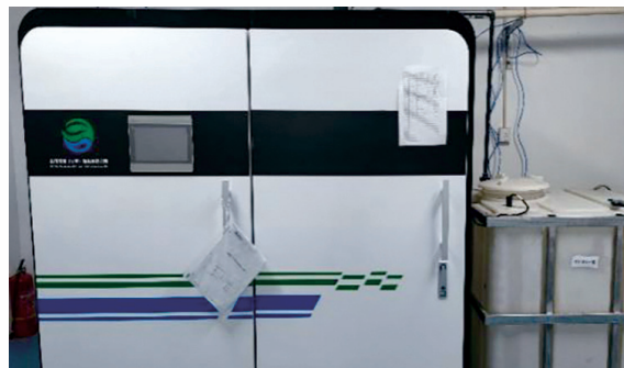
3D Medicines Beijing Laboratory sewage treatment device 思路迪北京實驗室污水處理裝置
