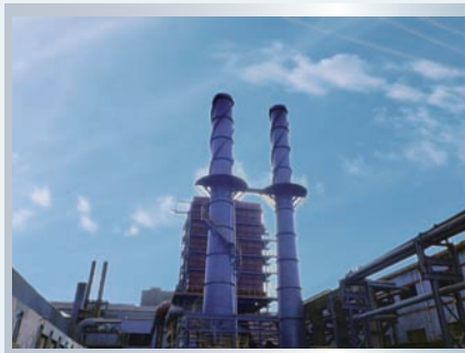
Strip steel plant heating furnace denitrification 帶鋼廠加熱爐脫硝
