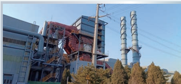
Section steel plant heating furnace denitrification 型鋼廠加熱爐脫硝
