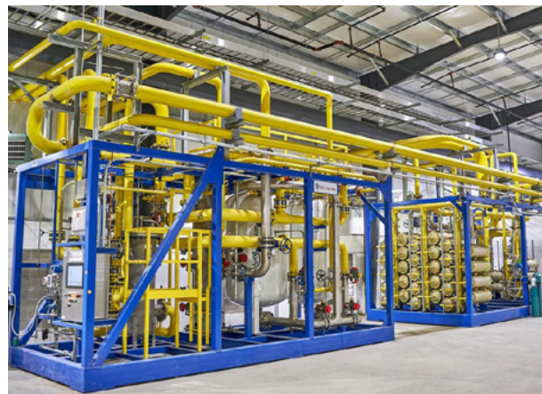
EDL's Wood Road RNG Facility in Michigan
