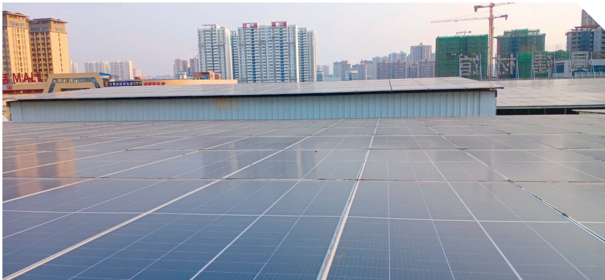
Photovoltaic power generation introduced in Nanning Dashanghui(南寧大商匯) project
