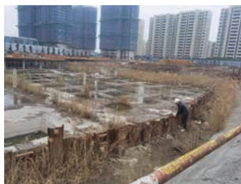
The Project Engineer is inspecting the retaining and protection for foundation excavation to ensure construction safety
