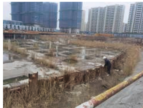
The Project Engineer is inspecting the retaining and protection for foundation excavation to ensure construction safety
