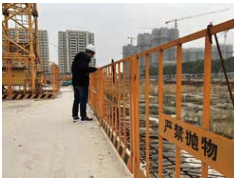
Inspection workers are examining whether the edge and opening protection is sufficient to ensure workers' safety
