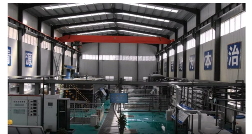
新疆天山胜利隧道生产废水处理厂 Xinjiang Tianshan Shengli Tunnel Production Wastewater Treatment Plant
