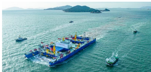
世界首艘自航式沉管运输安装一体船——“一航津安 1” The First Self-propelled Integrated Ship of Transportation and Installation of the Immersed Tubes in the World — "Yihang Jinan 1"
