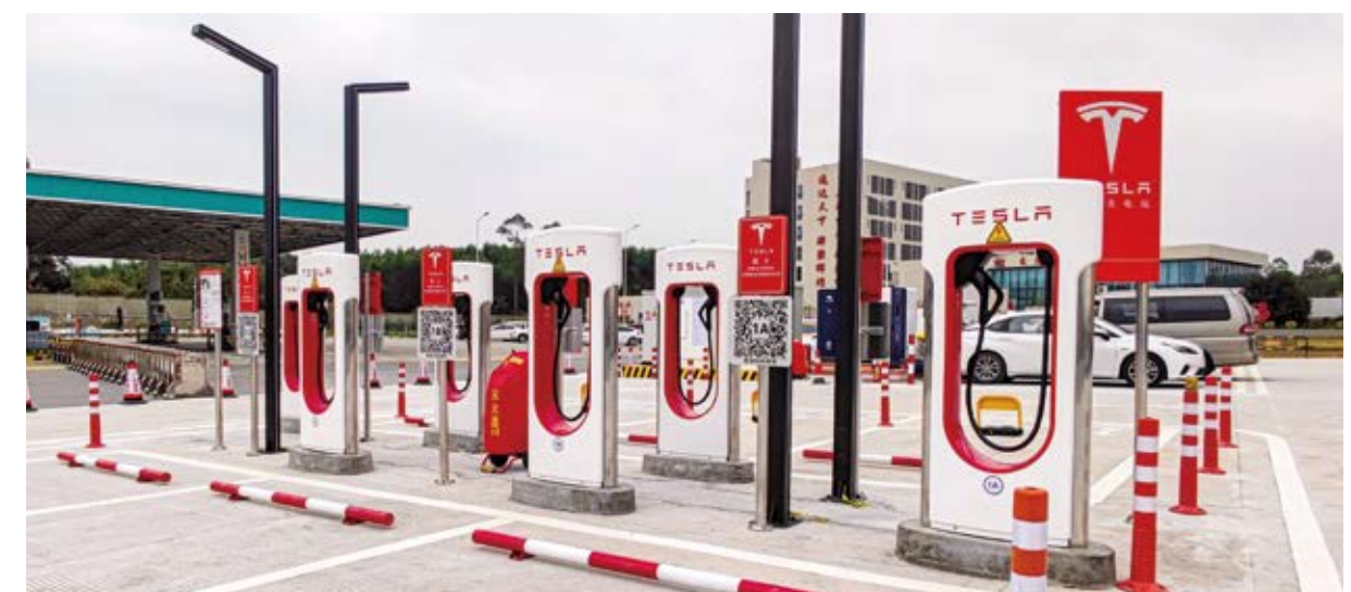
Tesla charging piles at Dahuai Service Area
