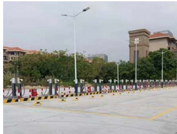
Yangjiang Public Bus Charging Station
