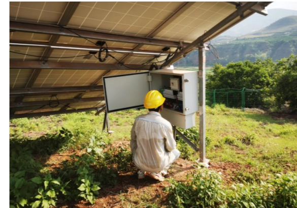
Photo: A staff on duty of a power station in Hewai, Yuanmou, Yunnan inspected the combiner box in PV array area.
