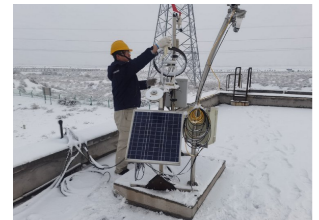
Photo: Emergency drill for extreme weather at Jingpu PV power station.
