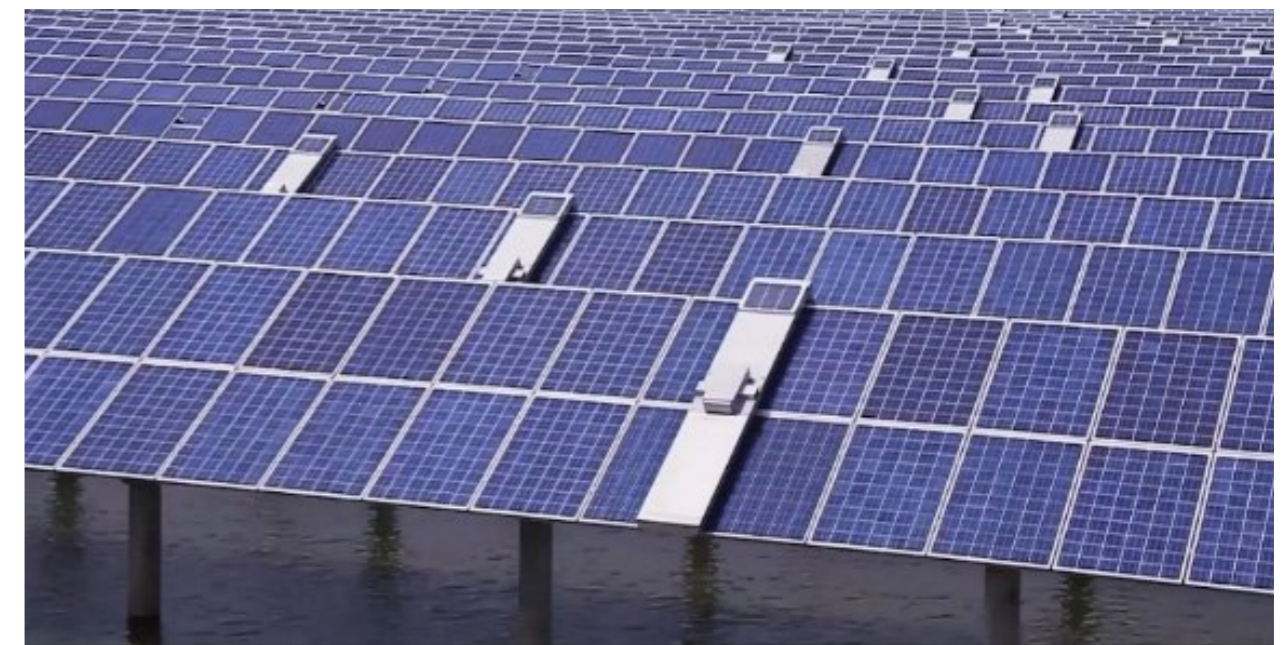
Photo: The Group's robot adoption in the operation and maintenance process has greatly reduced water consumption.
