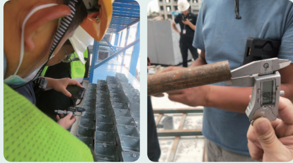
電盒壁厚、鋼管壁厚測量 Measuring the thickness of electrical boxes and steel pipes
