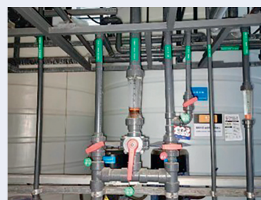
Recycled water pipes
