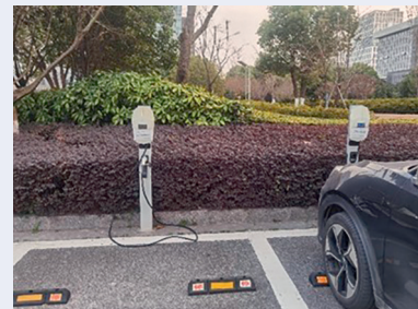
Charging piles for new energy electric vehicles
