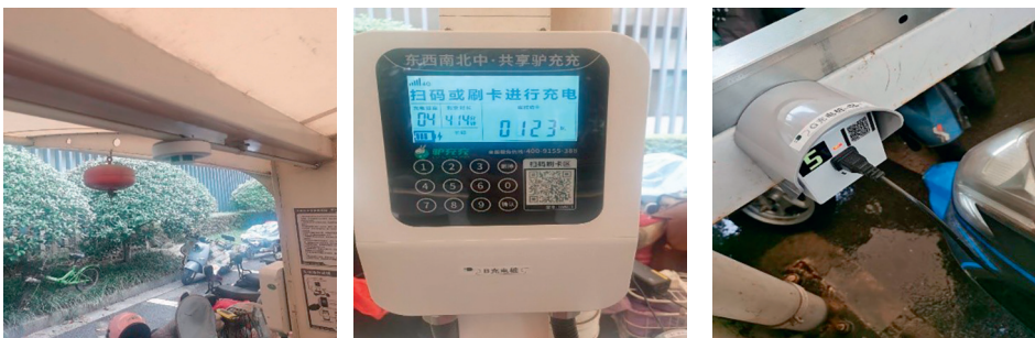
Smart firefighting facilities in the electric vehicle charging area
