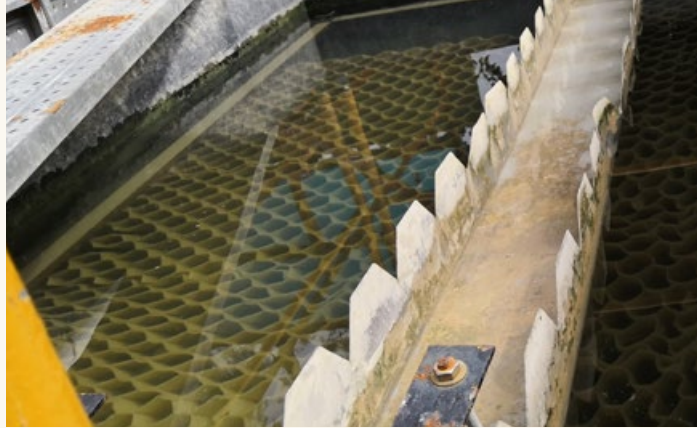
Waste water treatment plant
