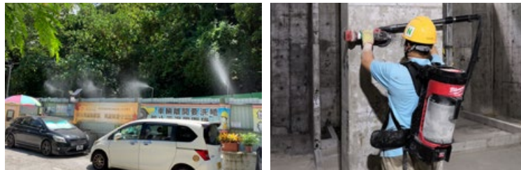
Automatic sprinkler system installed Grinder with dust collection
