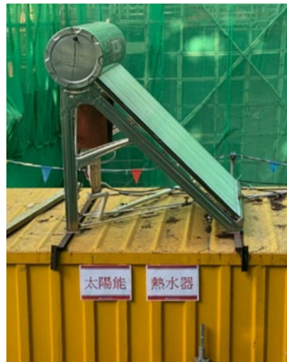
Water heater generated by solar power
