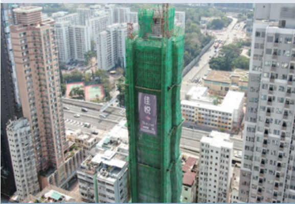
Haitan Street re-development project site at Sham Shui Po – The Vim 深水埗海壇街重建項目地盤—佳悅
