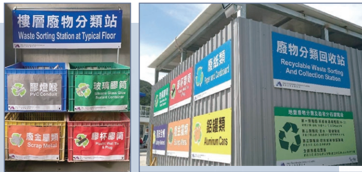
Set up waste sorting stations to improve cleanliness and tidiness of sites 設立廢物分類站，以改善地盤的整潔度
