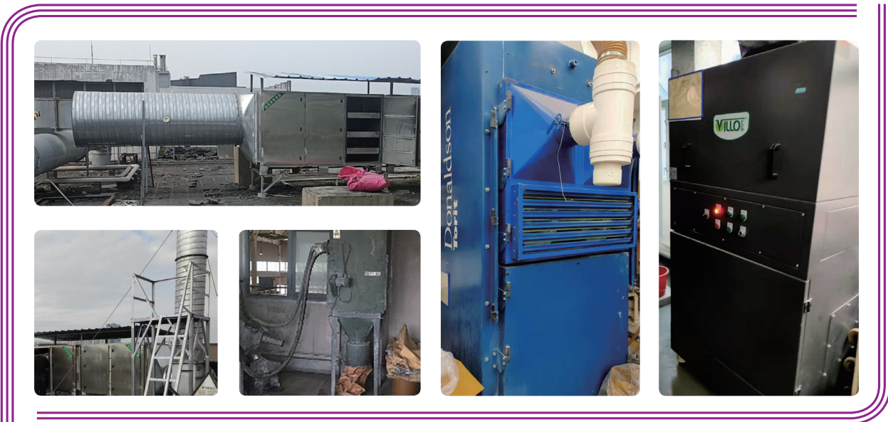
Exhaust air treatment facilities 廢氣處理設施
