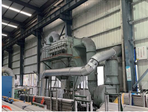
Production plants equipped with dust collectors with filter bags 生產廠房中設有布袋除塵器
