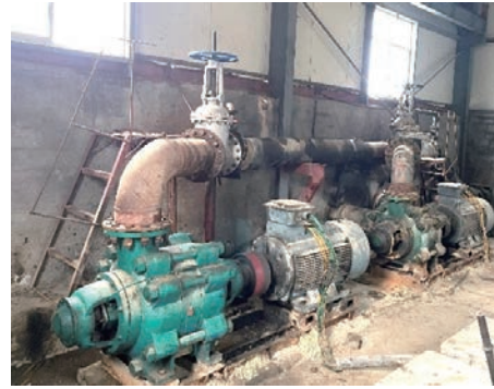
pump in pump station
