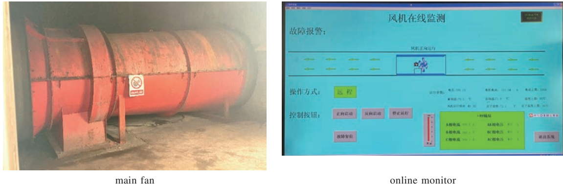
Figure 14-6: Main Fan at the Portal of Upcast
