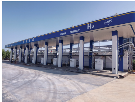
Hydrogen filling facilities in Jiyuan High-Tech Industrial Chemical Park
