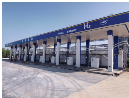
Hydrogen filling facilities in Jiyuan High-Tech Industrial Chemical Park
