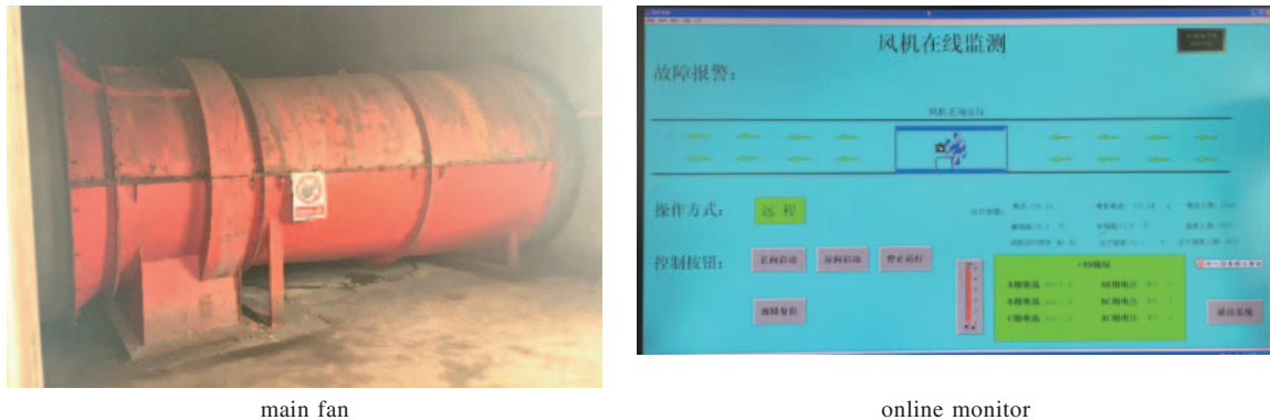
Figure 14-6: Main Fan at the Portal of Upcast
