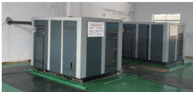
single screw air compressor
