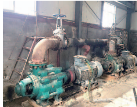
pump in pump station
