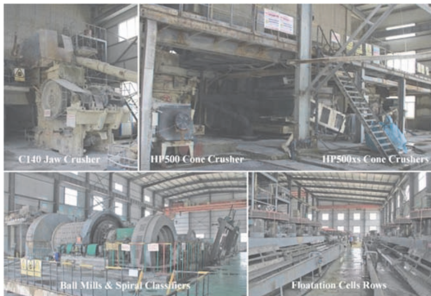
Figure 15-6: Photos of Processing Equipment
