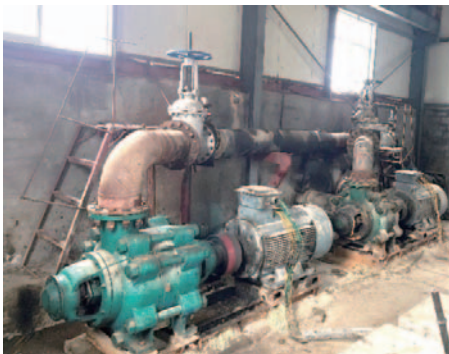
pump in pump station
