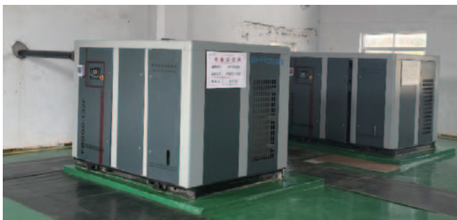
single screw air compressor
