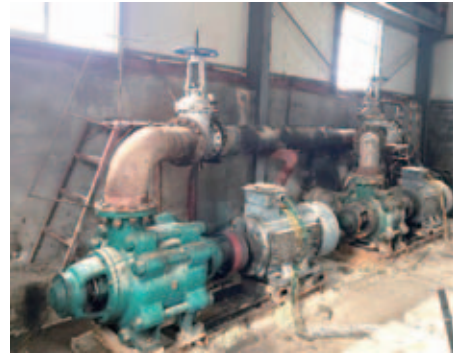
pump in pump station
