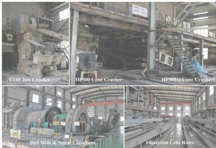
Figure 15-6: Photos of Processing Equipment
