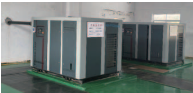
single screw air compressor
