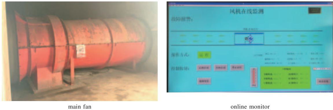
Figure 14-6: Main Fan at the Portal of Upcast
