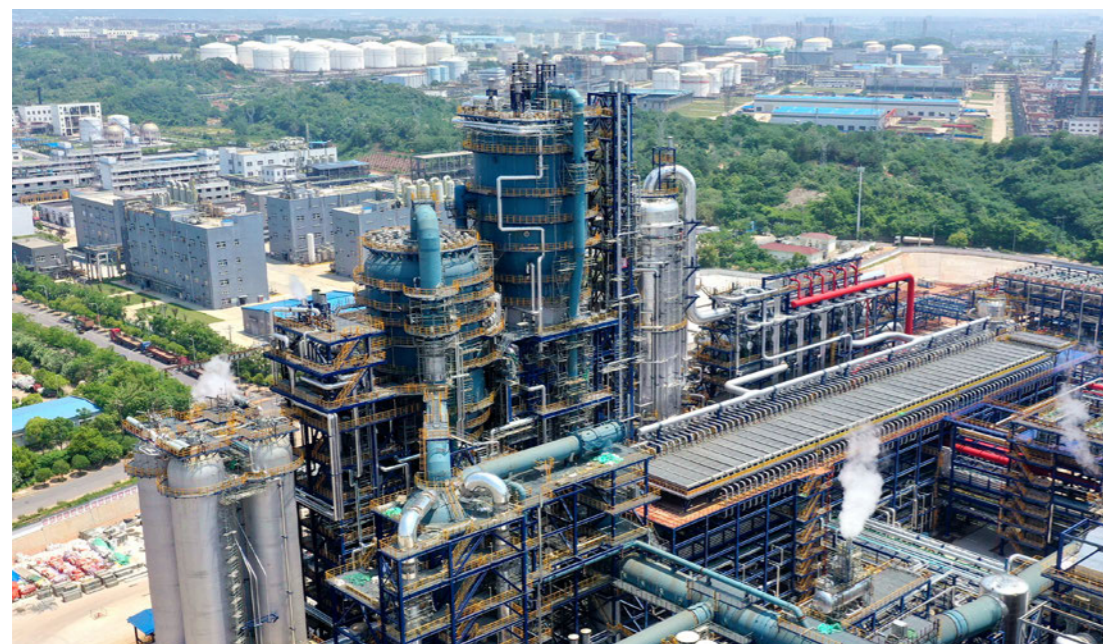
Heavy Oil Catalytic Residue Thermal Cracking Unit of Sinopec Anqing Petrochemical Company
