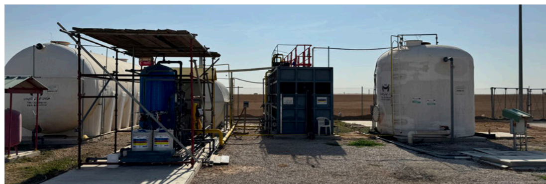
Sewage Treatment Equipment within the Camp
