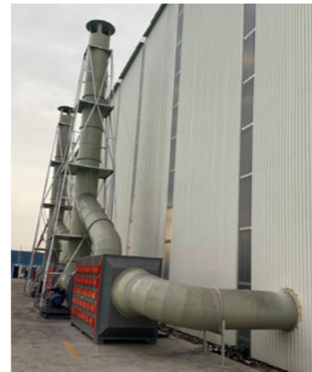
VOCs Gas Treatment Project
